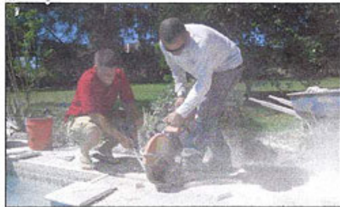
Jason Smith, left, owner of Outdoor Impressions, helps Nelson Borges cut paving installations for a pool deck in Valrico. The pavers come in a variety of colors, sizes and shapes, which Smith has customized to each job.
